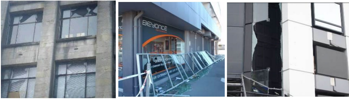
Figure 1. Examples of glazing damage that occurred in the September 4th 2010 Darfield earthquake (Dhakal 2010) and the February 22nd 2011 Christchurch earthquake (Baird et al. 2011).
