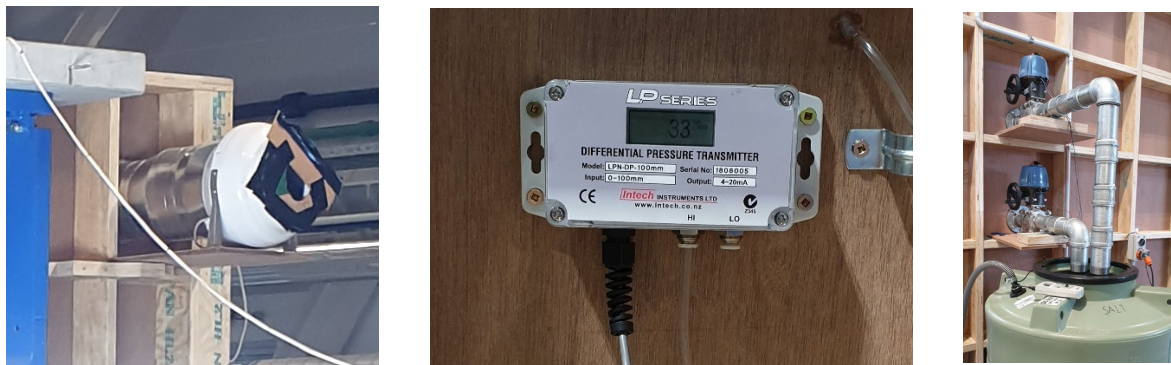
Figure 5. Air pressure control unit. Air blower (left), differential pressure sensor (middle) and bleeding valves (right).
