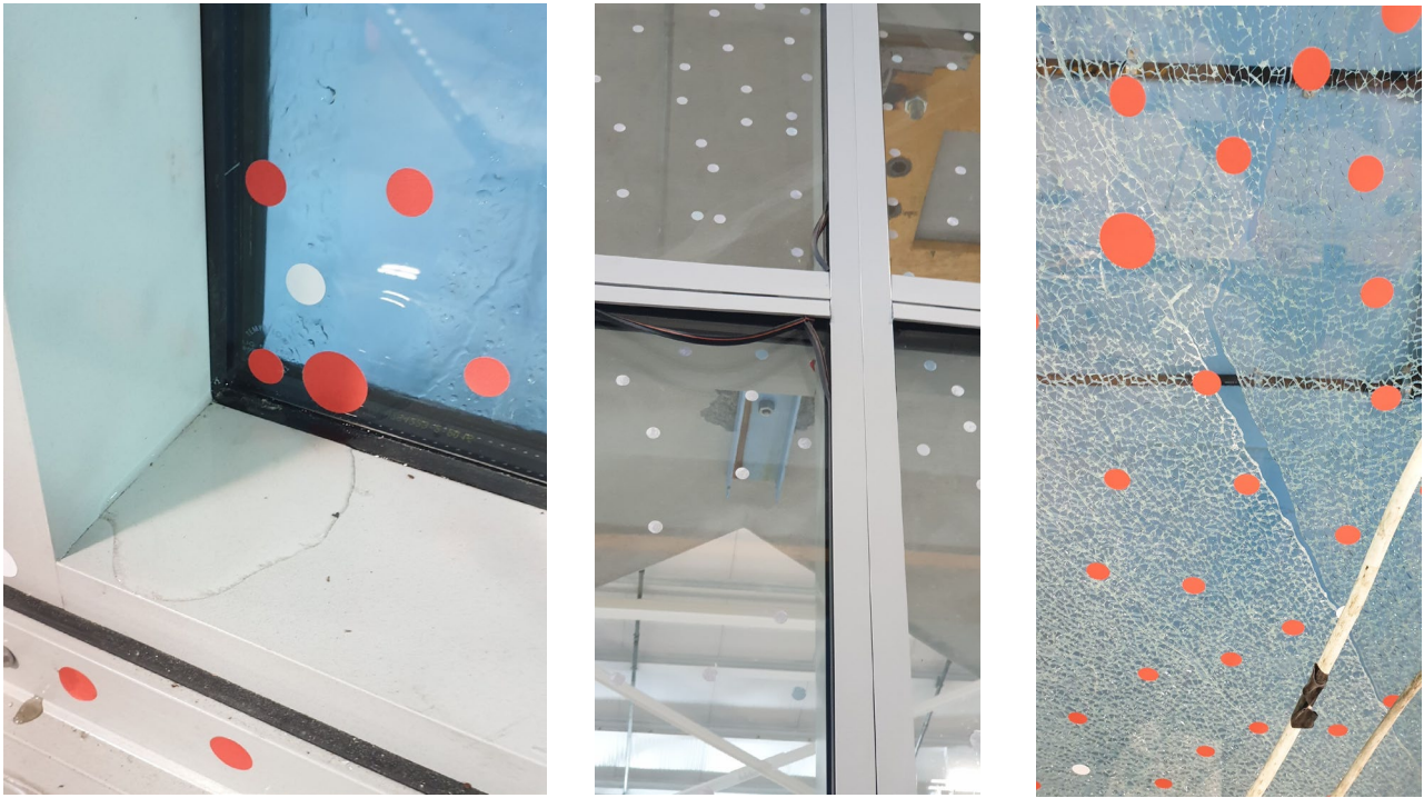
Figure 9. Damage states 1-water leakage(left), 2-gasket failure(middle) and 3-glass or frame failure(right).
