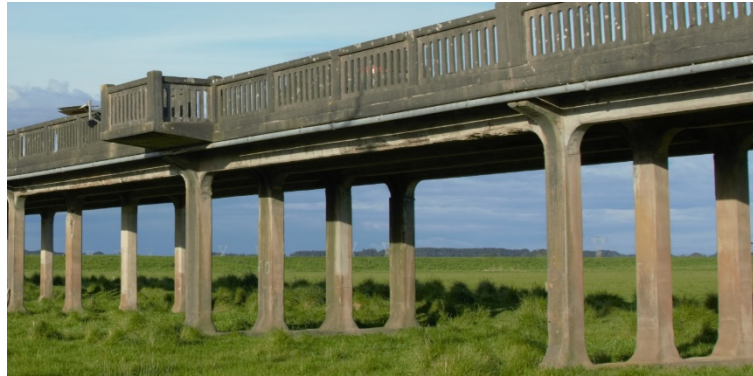
Figure 1: Side view of two spans of the Whirokino Trestle Bridge in Foxton, NZ.
