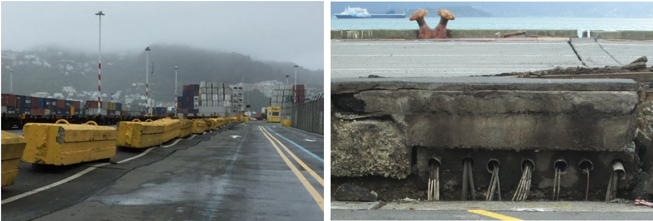
Figure 2: Some triage-stage observations: settlement, impact of buried structures, unstable containers, tilted light poles, exposed services, structural damage, operations on hold, ships at anchor.
