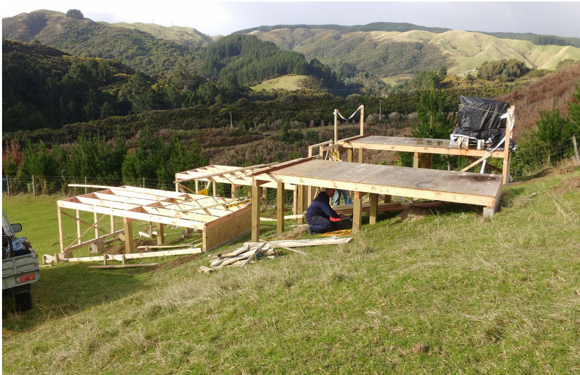
Figure 3: Photograph of overall set-up. NZS 3604 floors on right, pre-1960 floors on left.
