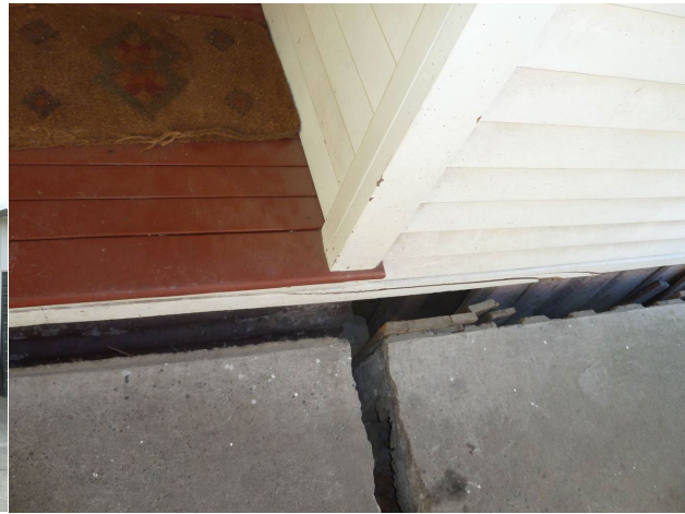
Figure 2: Downslope displacement of uphill foundation
