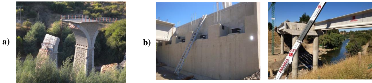
Figure 5: a) Rio Claro bridge collapsed in the 2010 Maule earthquake, b) Rio Claro bridge replacement using seismic isolation
