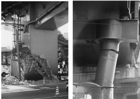
Figure 4: Damage and failure examples for bridges in the 1995 Kobe earthquake in Japan (Bruneau 1998)
