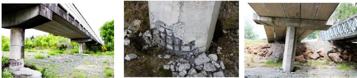
Figure 6: Damage examples for bridges in the 2016 Kaikoura earthquake in New Zealand (Palermo et al. 2017)
