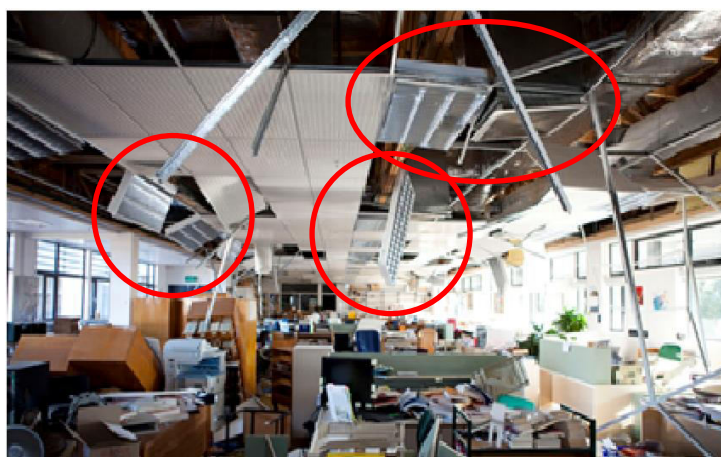
Figure 3 - Extensive damage to suspended ceilings in the Christchurch Earthquakes (MacRae et al. 2011)
