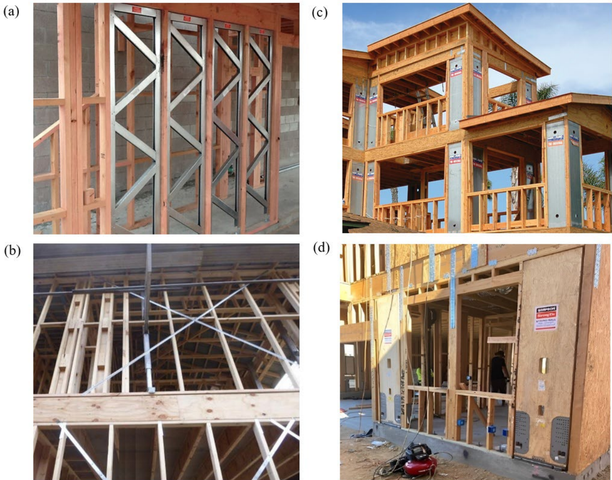
Fig. 2: Samples of seismic solutions for Residential applications: a) Truss bracing by Gamma brace Ltd., b) Tension-only straps, c) Steel shearwalls by Mitek Ltd., and d) Timber shearwalls by Simpson Strong-Tie Ltd.
