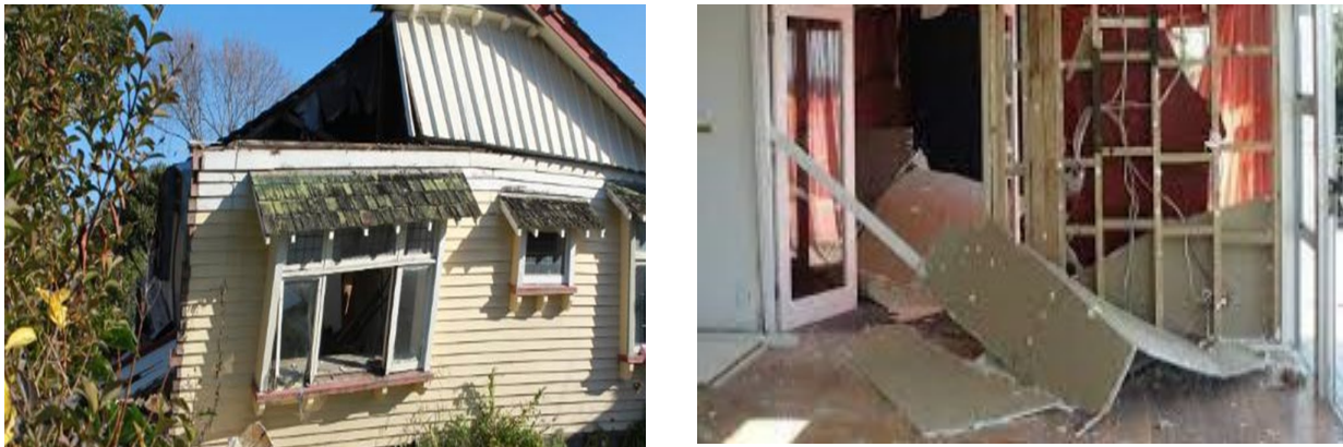
Fig. 1: Samples of seismic damage to residential buildings constructed by light timber framing
