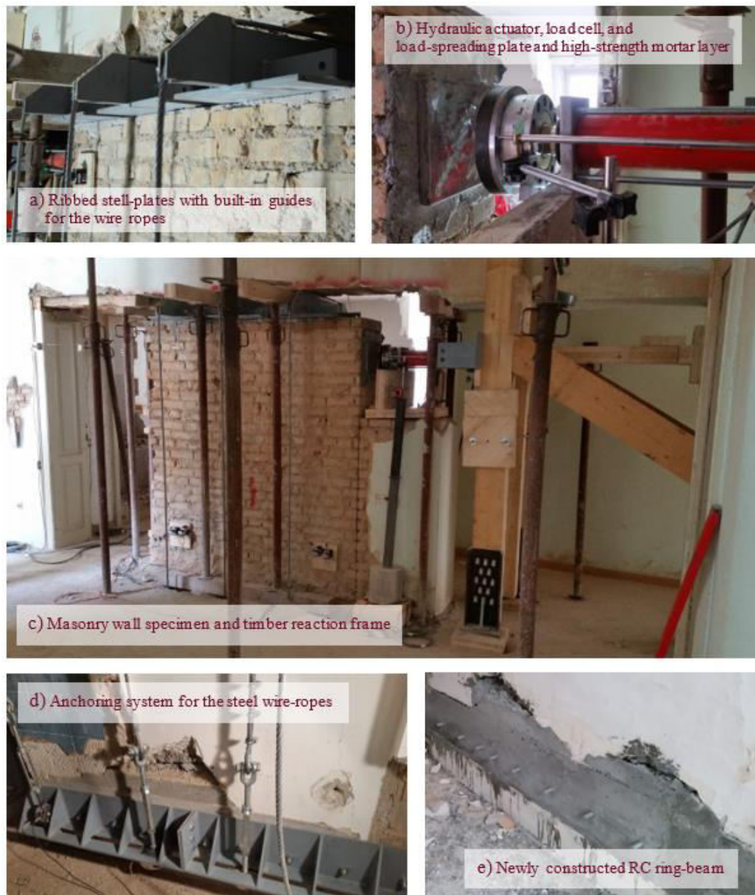
Figure 6: Details of the setup for the lateral testing of full-scale masonry shear walls
