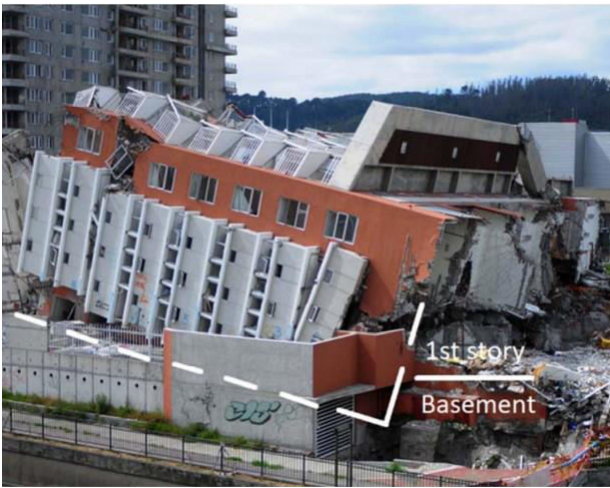
Figure 2: The Alto Rio building after the 2010 Maule, Chile Earthquake (Song et al., 2012)
