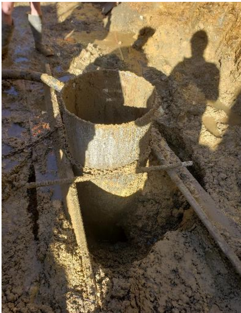
Figure 6: Case pile in collapsed hole
